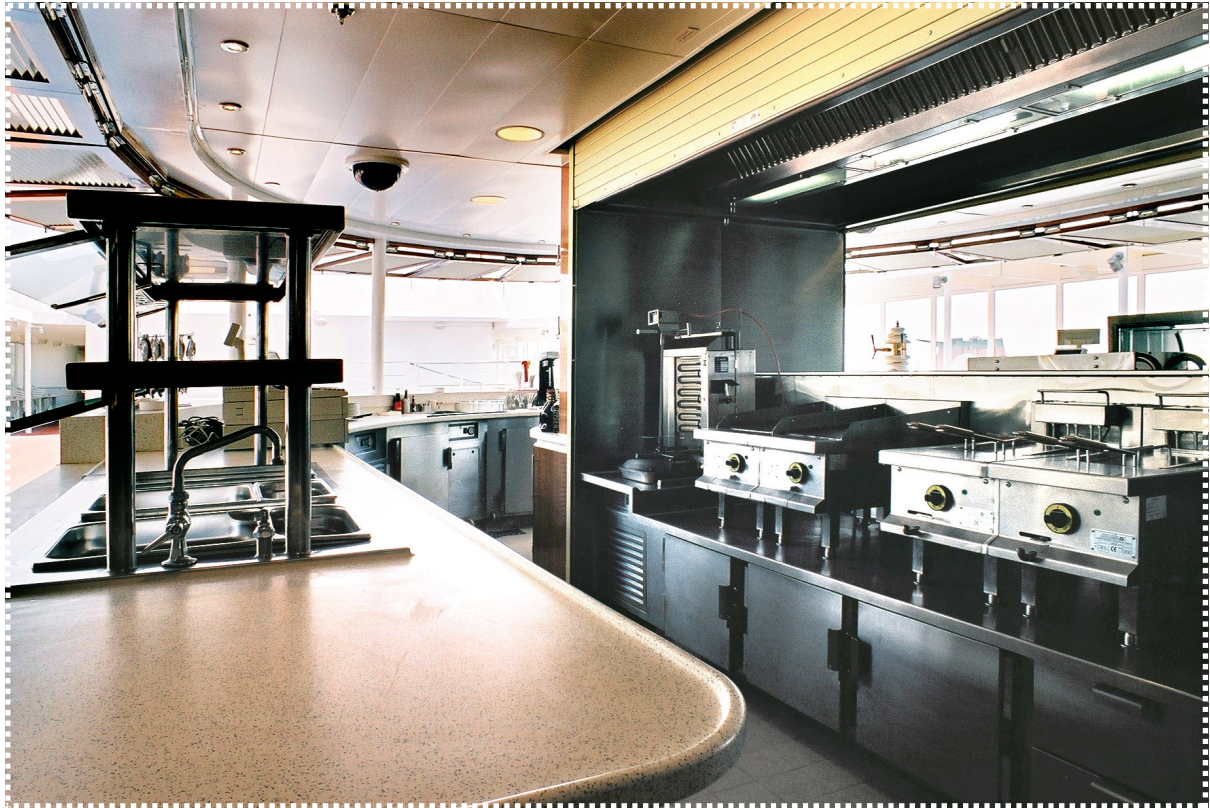
Outside bar showing a pair of table top griddles and table top fryers built in stainless steel
